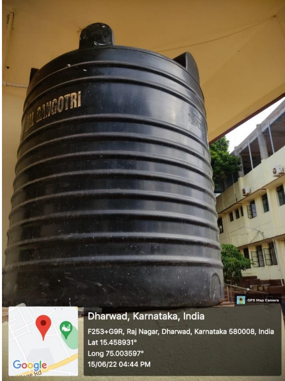
WATER TANK INSTALLED IN COLLEGE
